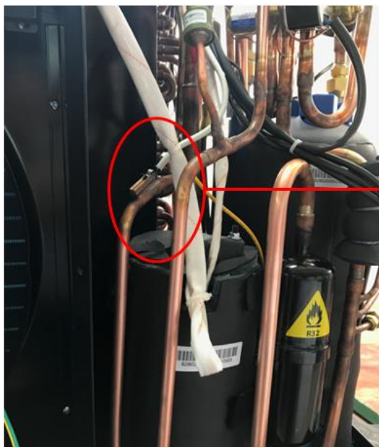
Gas exhaust temp sensor position: On gas exhaust copper pipe
